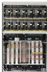
Power cell cabinet (Top) Transformer cabinet (bottom)
